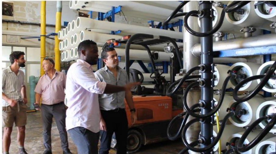
Site visit to the Għar Lapsi Desalination Plant in Malta as part of a Short-Term Scientific Mission (STSM)
