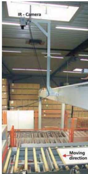
Figure 6.4: Set-up for passive thermography behind the press.
