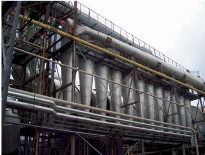
Figure 3.2: Dryer in a particleboard plant (Sonae Indústria, Oliveira do Hospital plant).
