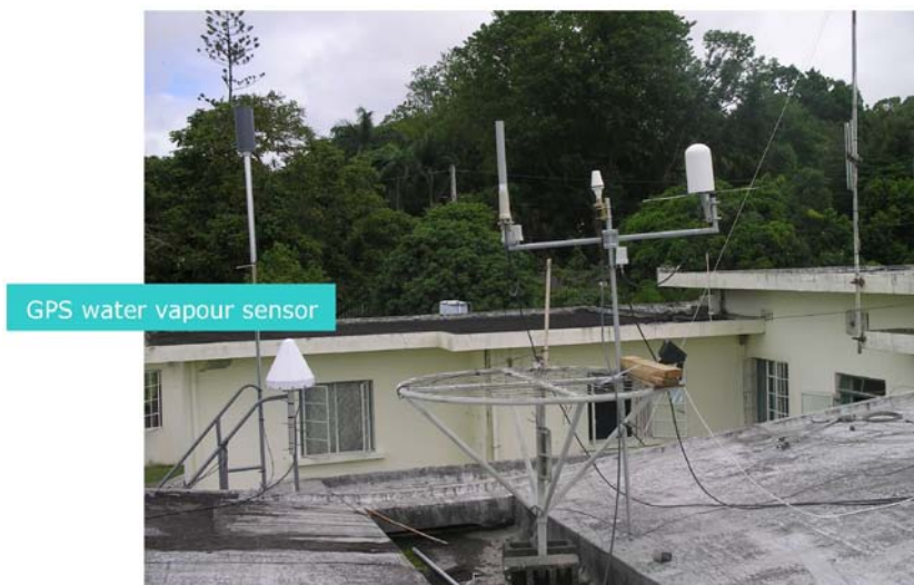
Figure 5.43. GPS water vapour sensor installed on the handrails of the staircase to the roof, Vacoas
