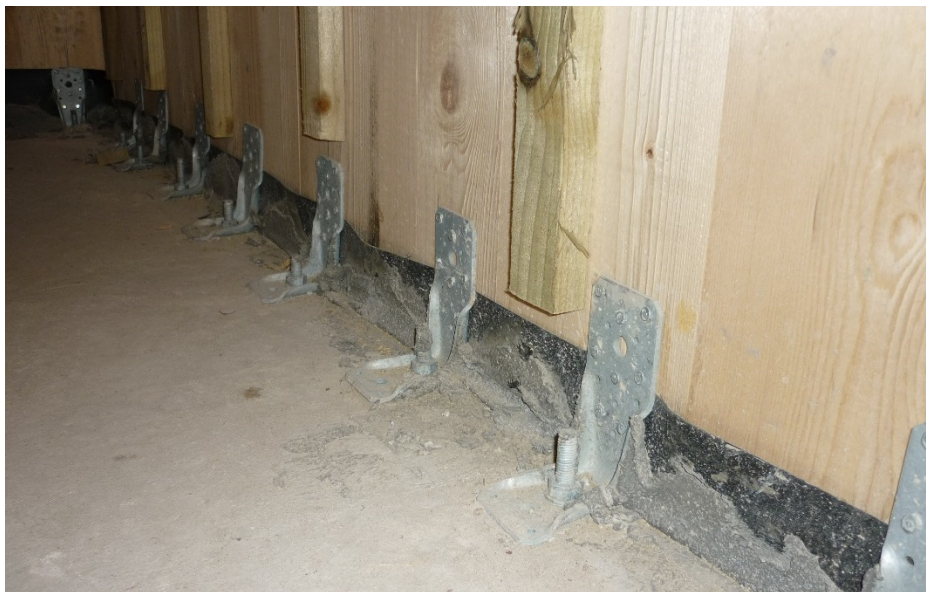
Fig. 9 Typical CLT wall to concrete connection with grouted gap at wall base.
