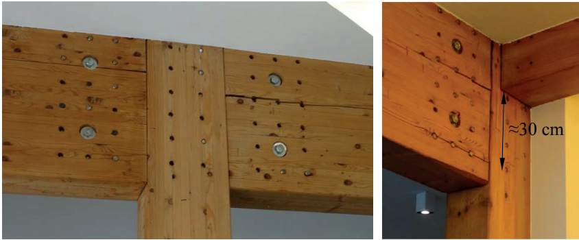
Fig. 5 Appearance of shrinkage cracks in the area of a flitch plate dowel - rigid connection in very dry conditions
