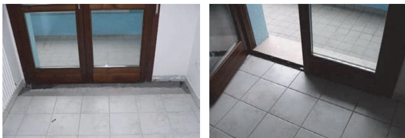
Figure 10.5. View of the French window area with the first row of tiles and floating mortar removed (on the left) and after the repair (on the right).
