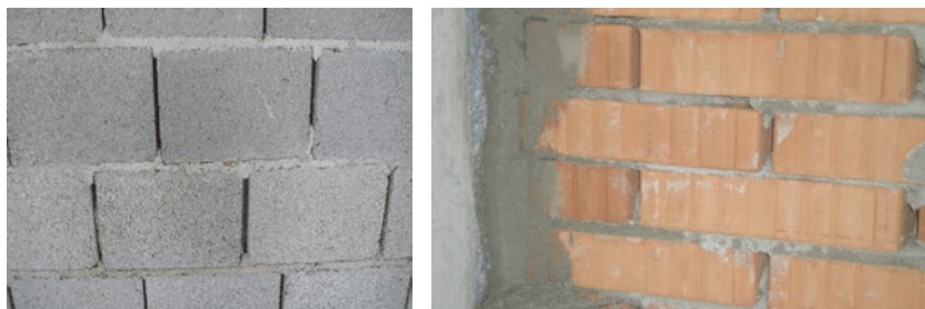
Figure 10.4. Examples of lack of mortar in vertical joints between blockwork.
