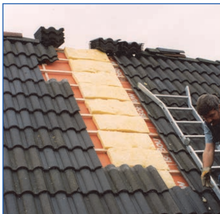
Figure 10.29. No mineral wool sound barrier above partition wall in combination with roof elements with rigid thermal insulation (PUR, PIR, EPS) leads to a decrease of 5 – 10 dB in airborne sound insulation between rooms.
