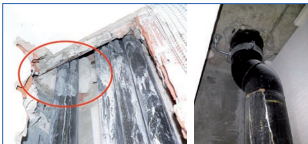
Figure 10.9. Waste water pipes embedded in mortar (left). Changes of direction in waste water pipes (right).
