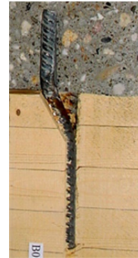
b.) example of a failure mode
